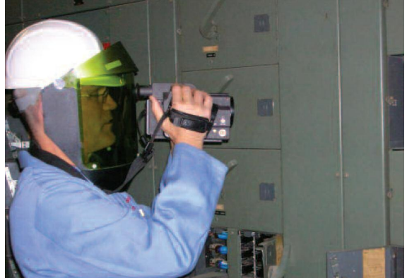
Infrared thermographers look for hot spots that could indicate loose connections and other electrical problems.
