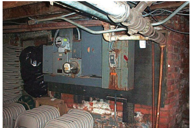
Electrical equipment rooms used for storage create property and liability exposures.
